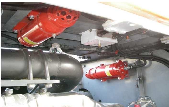
Fig. 2. Powder fire extinguishing module
